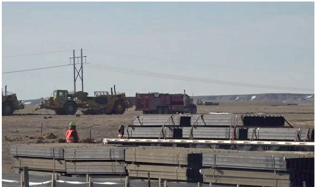
Construction began earlier this year on a large solar farm near New Underwood in Pennington County. Some of the power will be purchased by Basin Electric and be distributed to cooperatives in South Dakota.
