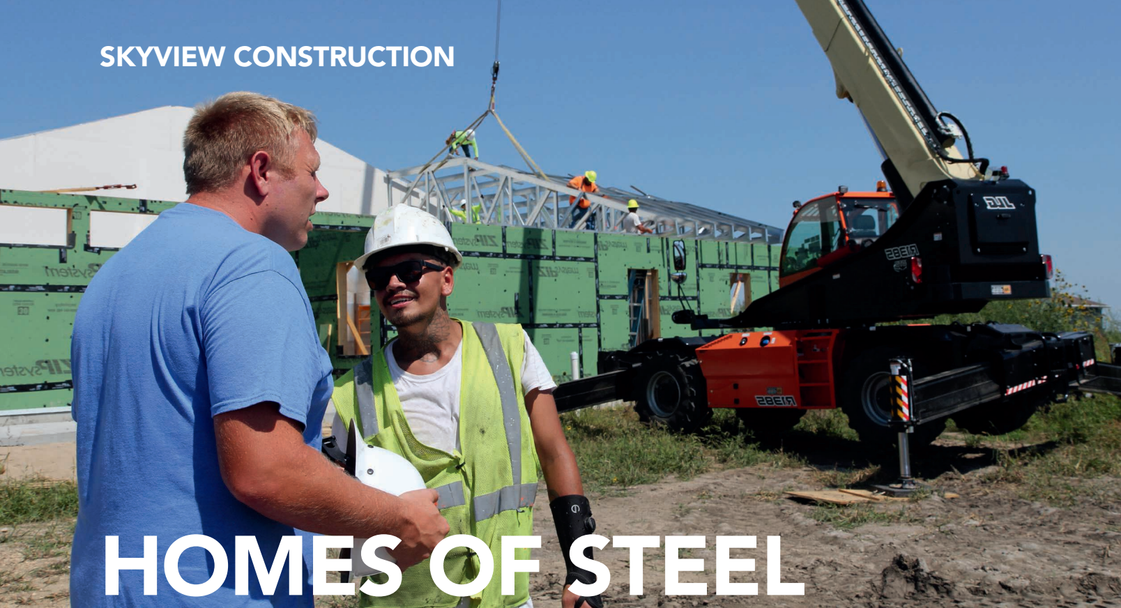
Mike Adolph, left, checks in with an employee during a break from construction on Aug. 22 in Watertown. Photo by Shannon Marvel
